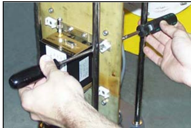
Removing/attaching radio modem
