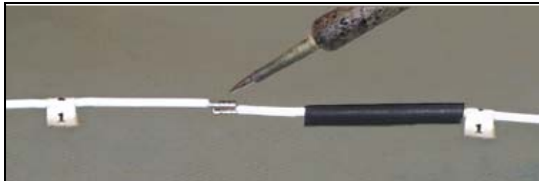
Solder the wire labeled 1 on the new connector to the wire labeled 1 from the old bulk head connector
