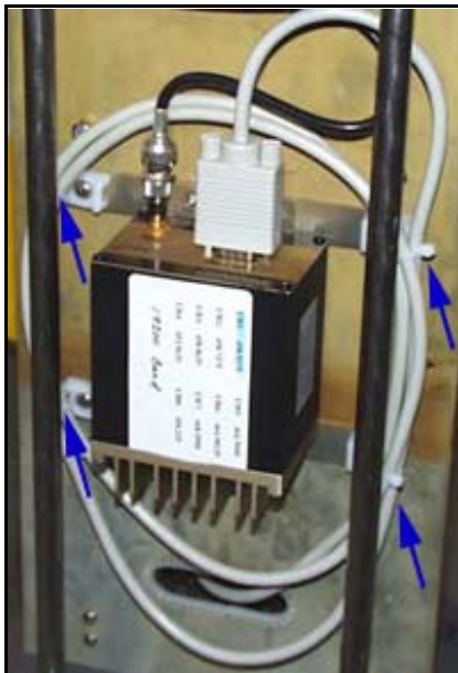
Locations of cable ties and position of cable and radio modem
